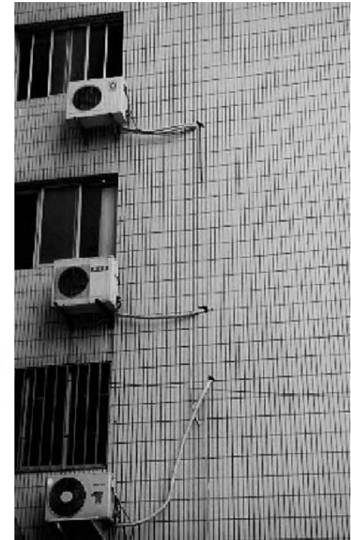
Figure 14 Image of residential building with unsealed through-wall piping from air-conditioning units
