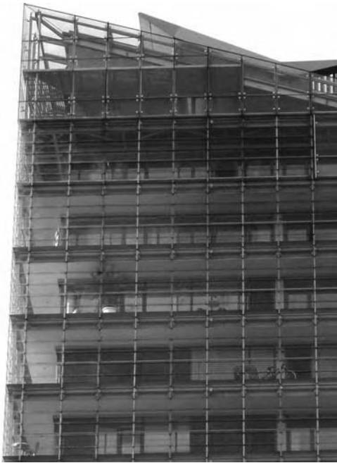
Figure 17 Double-skin glass louvered façade for an apartment building in Manchester, U.K. (architect: Ian Simpson Architects)
